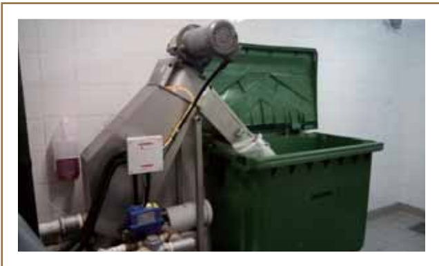
The new Hobart Pulper food waste handling machine installed at the team members' canteen at Galaxy Macau™ Phase 2 greatly reduces the food waste volume by 80% through compression and dehydration
